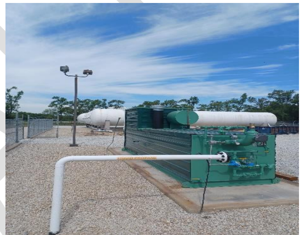
Peak Shaving Plant
